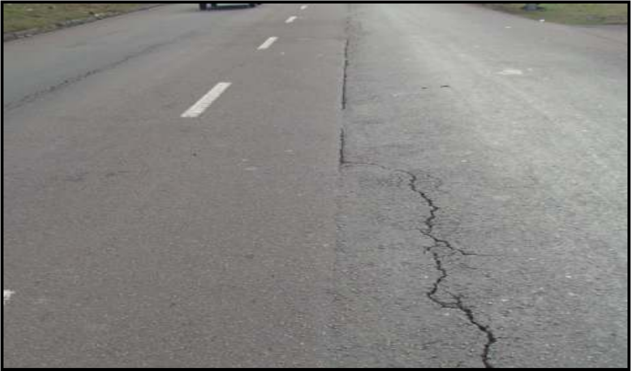
Figure 3: Longitudinal cracks on Bayhead Road
