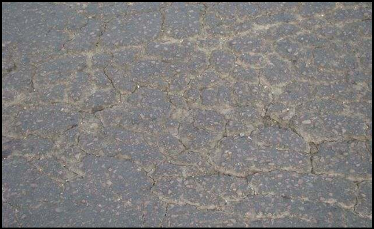
Figure 2: Crocodile cracks on Maydon Road
