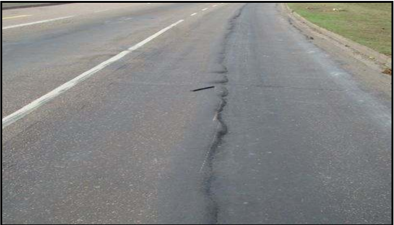
Figure 4: Depression on the asphalt layer on Bayhead Road
